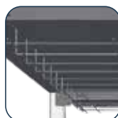
Horizontal Cable Duct
